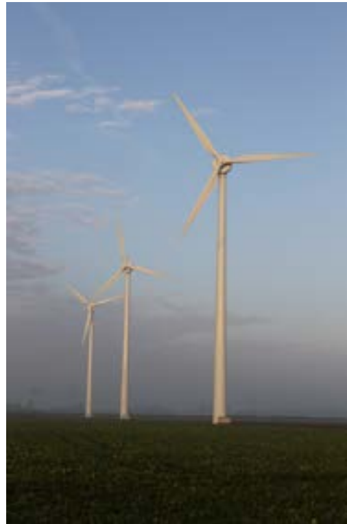
EWT DW 54 / 900 kW Wind Turbine
